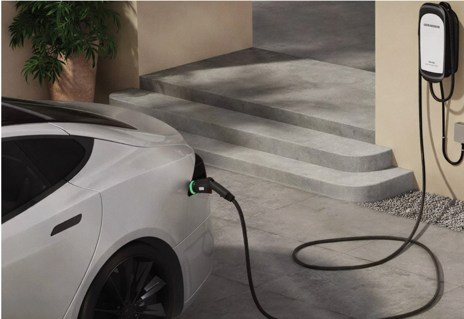
Provision of EV charging station
